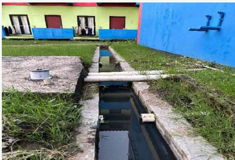
Retention pond system — campus wastewater management & natural sedimentation
