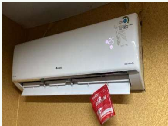
Air Conditioning units across campus buildings (394 units total)
