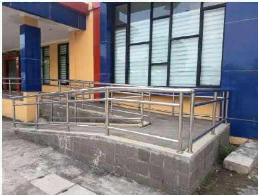
Disability ramp with stainless steel handrails
