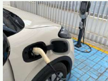
Electric Vehicle Charging Station — dedicated EV charging infrastructure on campus
