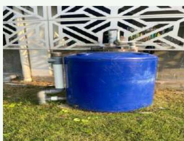
Rainwater harvesting — HDPE Penguin-brand tanks with PVC piping
