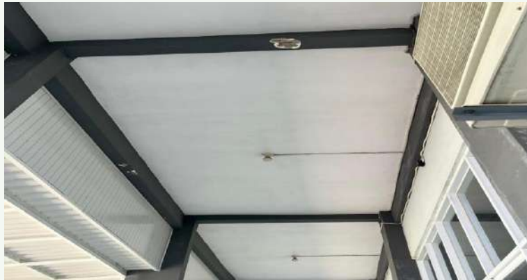
LED lighting panels installed on ceilings across campus buildings — 72.3% LED coverage (4,075 of 5,633 lamps)
